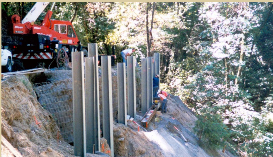
Construction of sliver fills is a complicated, technical task, often involving limited site access.
