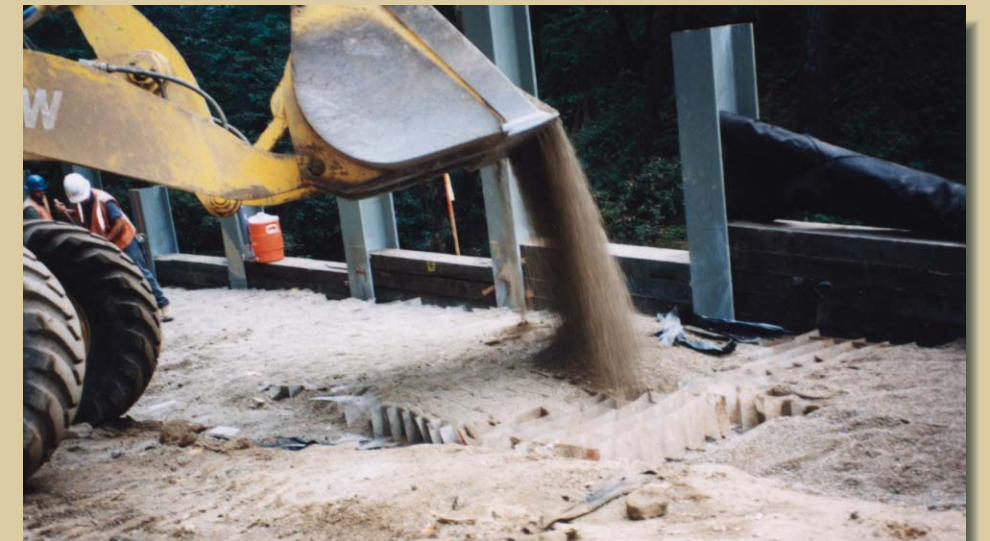
Building trafficable surfaces using geocellular materials is a well-understood and well-documented practice.
