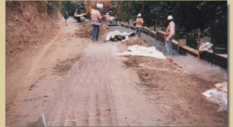
RDFW was used in road shoulder construction. Confined-cell geosynthetics (geocells) can provide the same load-bearing strength as much thicker rock-filled base.
