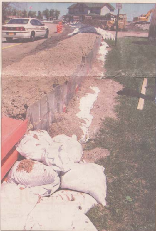
▲ This 4,400-foot-long dike, built to protect Warroad, Minn., from Lake of the Woods, uses three types of material.
